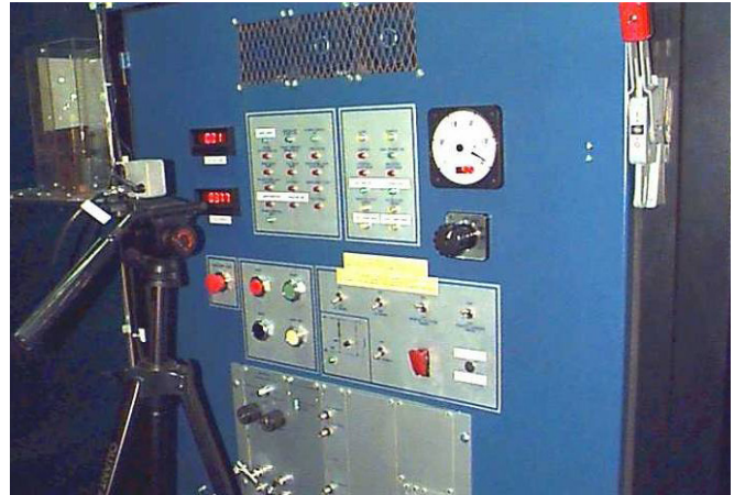
FIG 1. Dynapower magnet power supply.
